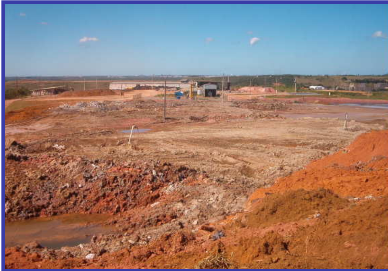
Landfill before the implementation of a landfill gas capture and utilisation system
