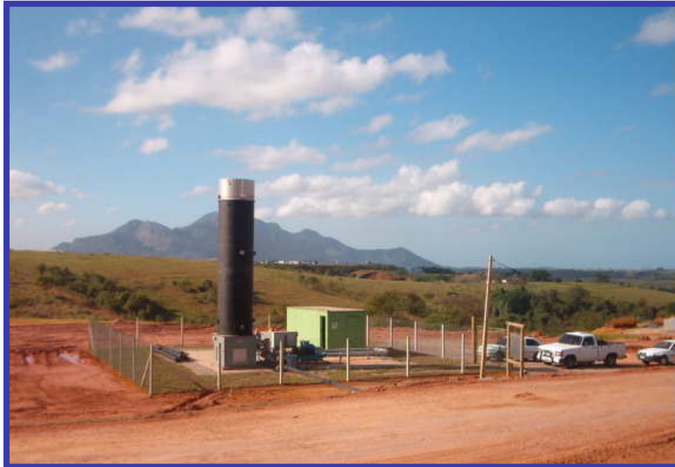
Landfill gas flare system installed
