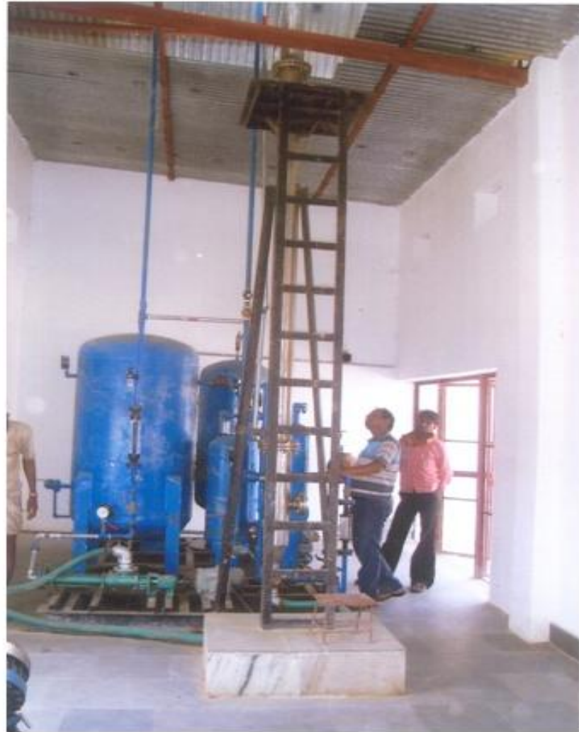
Biogas Enrichment Plant
