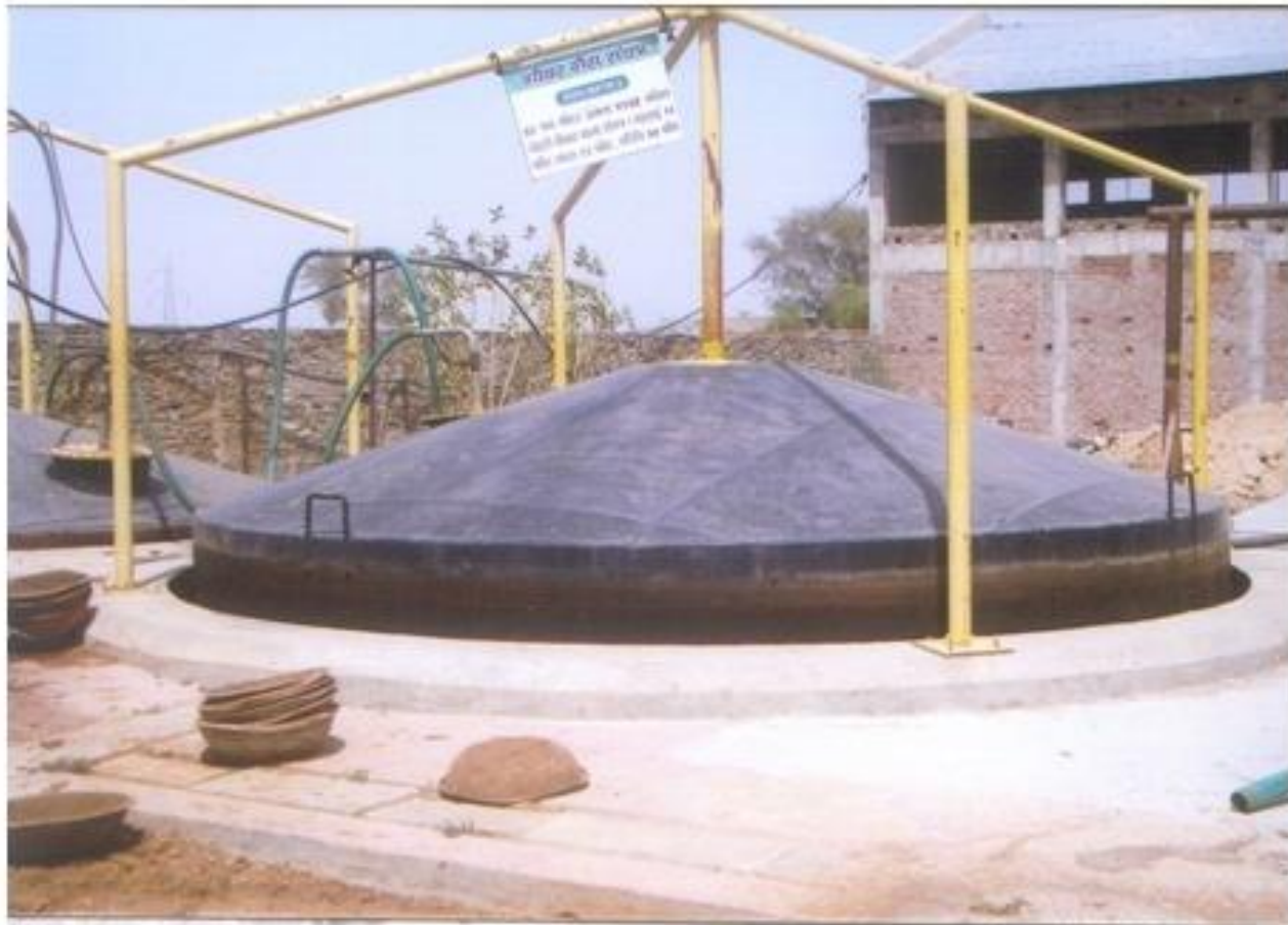
Biogas Plant at Bhilwara Gaushala
